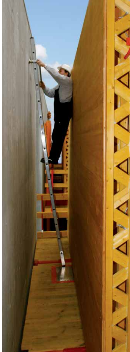
Safe working conditions on the CB 240 in protection of the formwork element.
