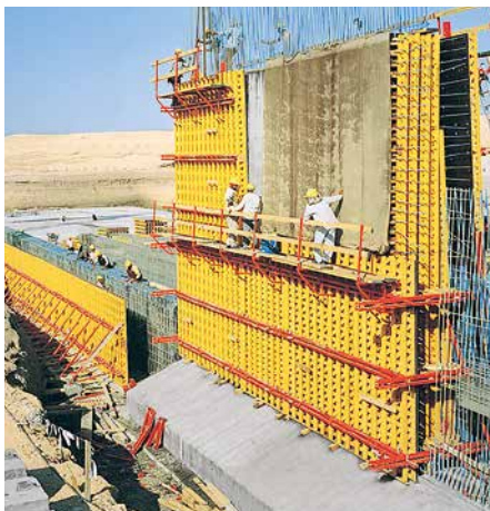
VARIO GT 24 being used to build a sewage treatment facility with tapered walls.
