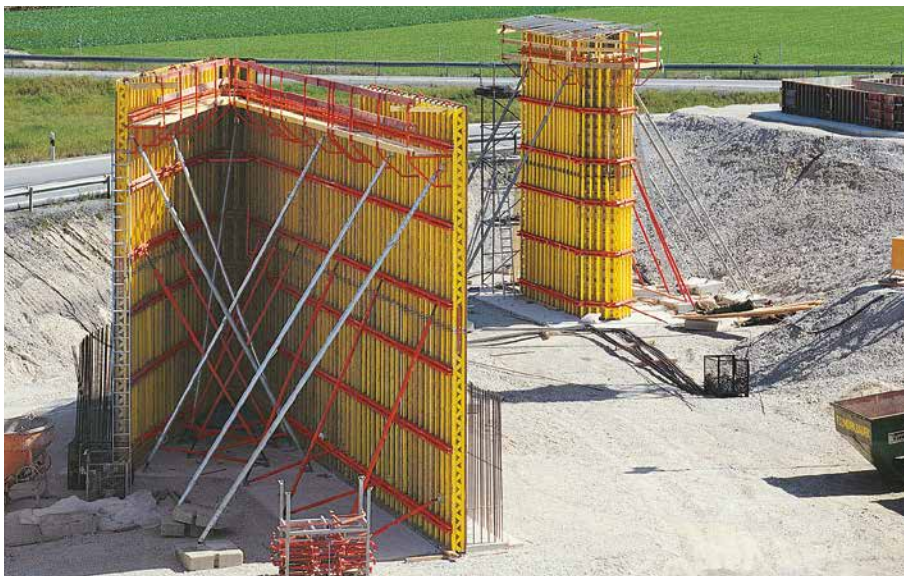
Abutment and bridge pier with VARIO GT 24. Crossing structure for the suburban railway line to the new Munich Airport.
